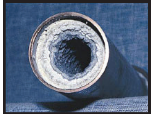
2A A 2 in. diameter copper pipe lined with about 1 in. of scale.
